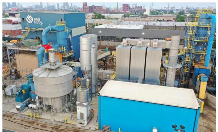
New advanced emissions capture and control system, now online at Sims Metal in Pilsen
